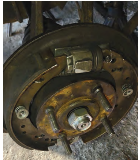
15. The hub/vertical link assembly held on the shaft with the axle nut.
